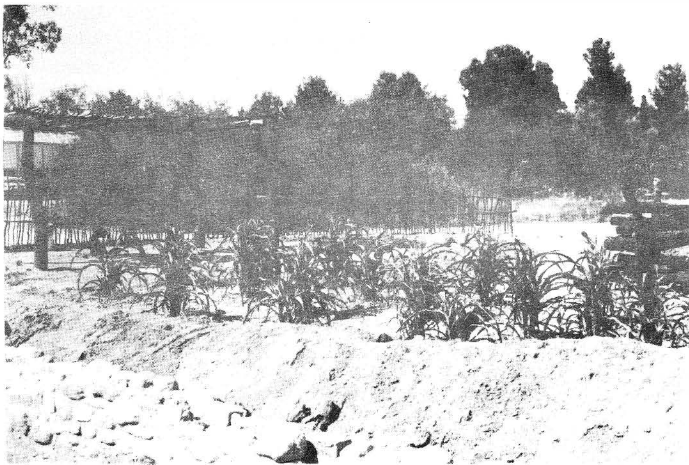
The new garden is shown here during construction this July. In the foreground is the Hopi terrace and piled earth ready to be shaped. The floodwater field, ramada and ocotillo fence are in the background.
